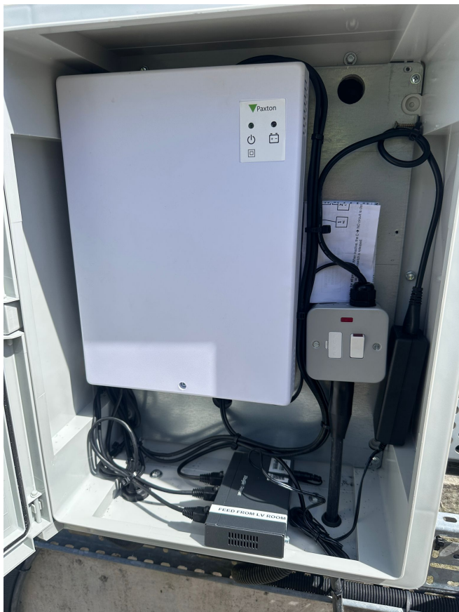
Switch and power location image
